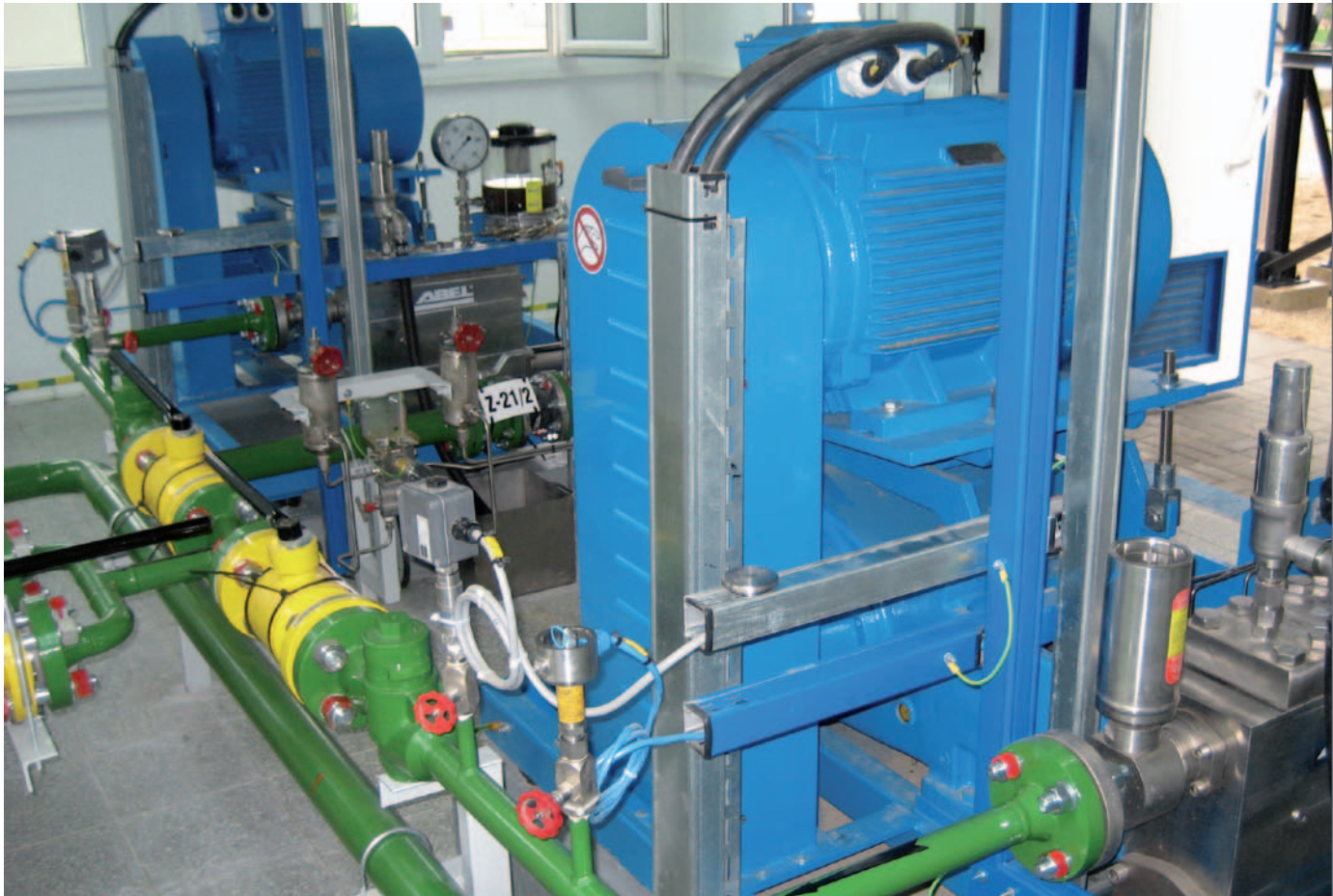
ABEL HPT for injection of oily brine water for gas extraction
