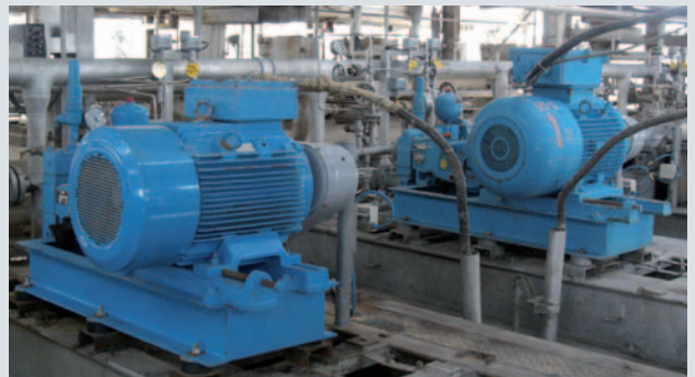
ABEL high pressure pump for injection of ethylene in gas drying process
