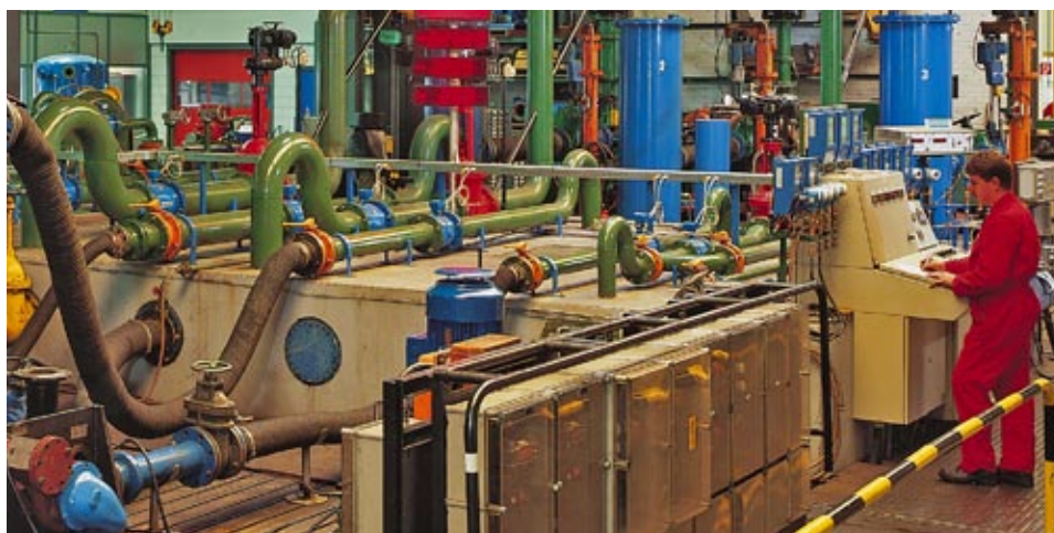
Test bed Johnson Pump in Assen
