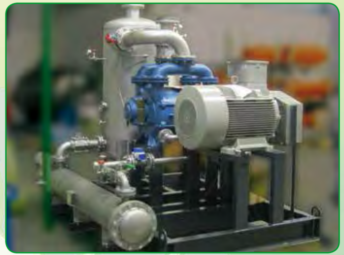
Vacuum units for biomasses co-generation plants
