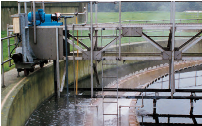
Wastewater treatment is a difficult pumping application that Hydra-Cell routinely handles.
